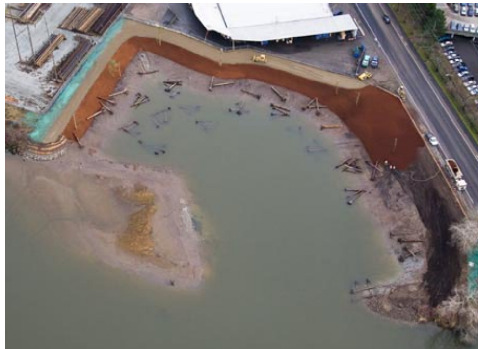
Installation of rootwads and anchors along the Estuarine Reach of the Duwamish River
